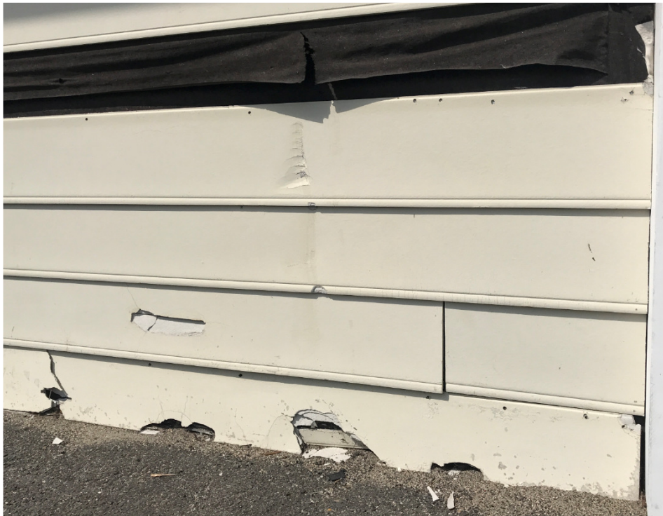
Pictured: Fiber cement siding impacted in various ways on a commercial building
