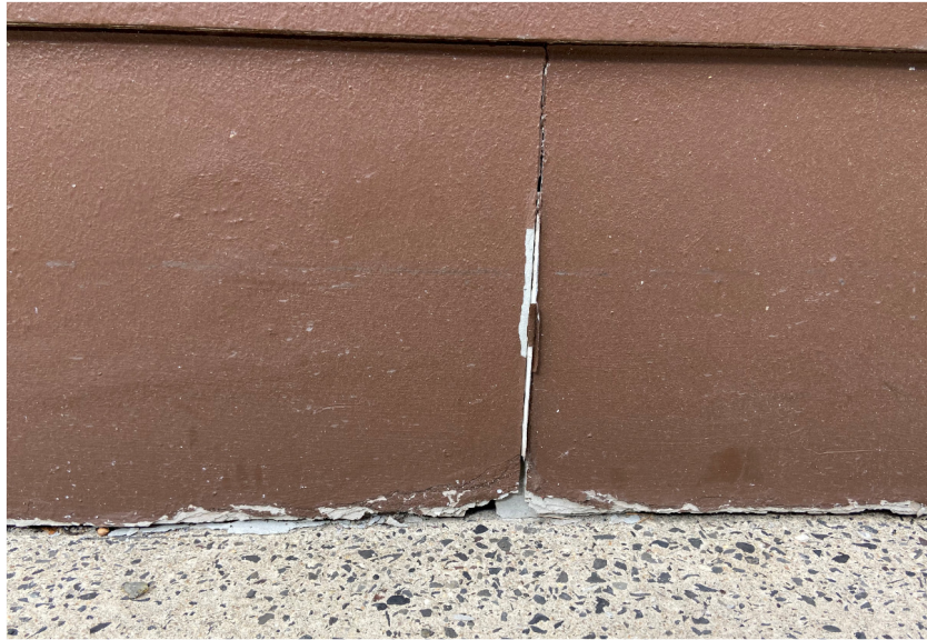
Pictured: James Hardie installed too close to grade and immediately failing
